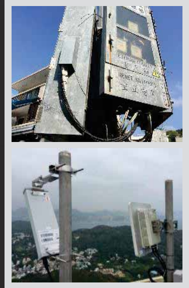
Hong Kong Electric, Hong Kong
